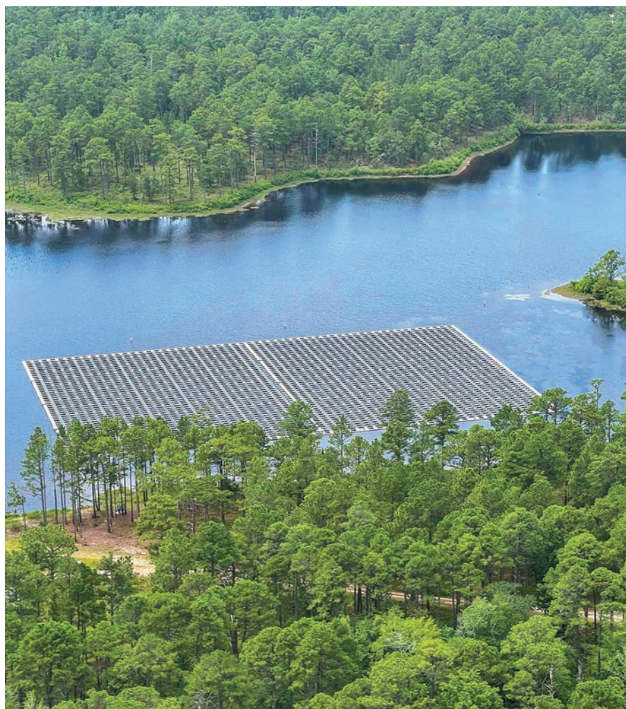
Floating solar microgrid consisting of 2,700 solar panels on lake at nearby Camp Mackall provides clean energy to Fort Liberty, North Carolina, July 28, 2023 (U.S. Army/Jason Ragucci)
