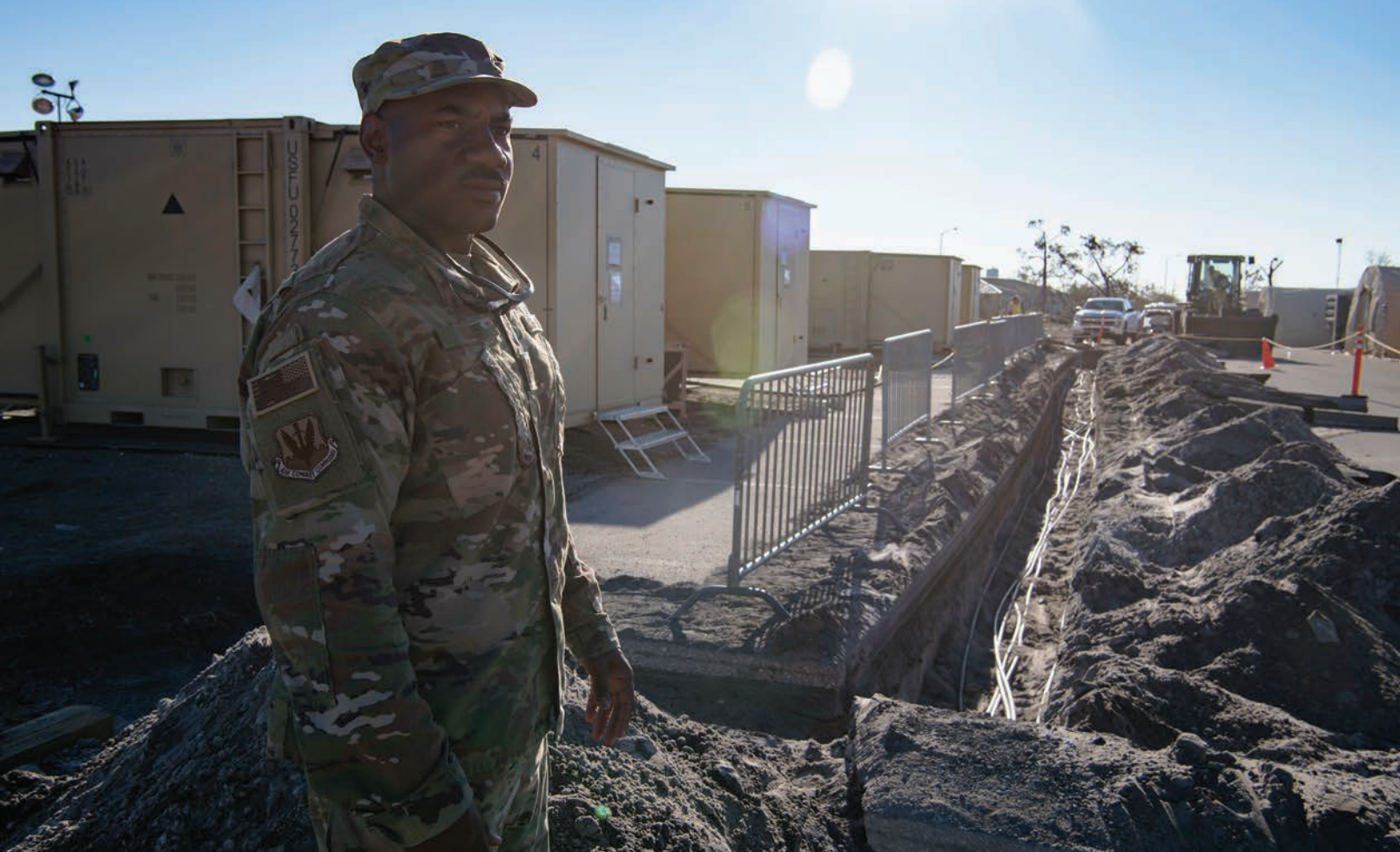
Technical Sergeant Marquelle Willis, 23 rd Civil Engineering Squadron, Moody Air Force Base, Georgia, Prime BEEF, electrical systems noncommissioned officer in charge, works to repair high-voltage power lines supplying electricity to tent city, Tyndall Air Force Base, Florida, October 28, 2018, after Hurricane Michael (U.S. Air Force/Kelly Walker)
